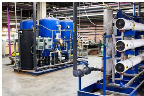
SJSU reverse-osmosis equipment for steam make-up water.
