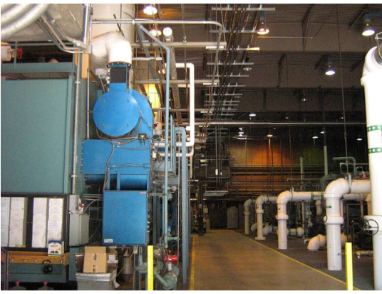
SJSU central plant.
