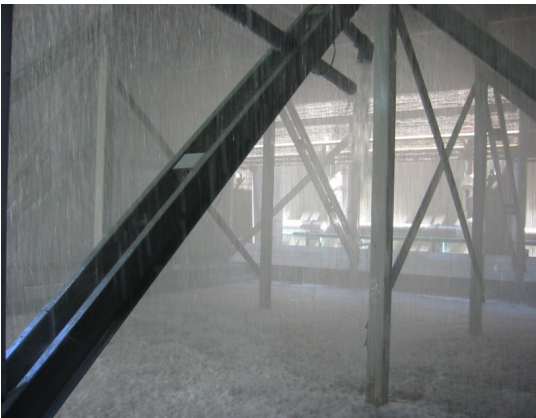
SJSU cooling towers
