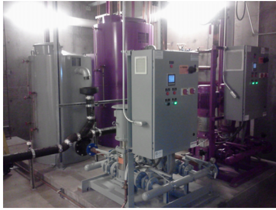
SJSU King Library indoor recycled-water equipment.
