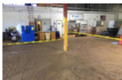
The support column was deemed structurally unsound resulting in a 50-foot radius being cordoned off.
