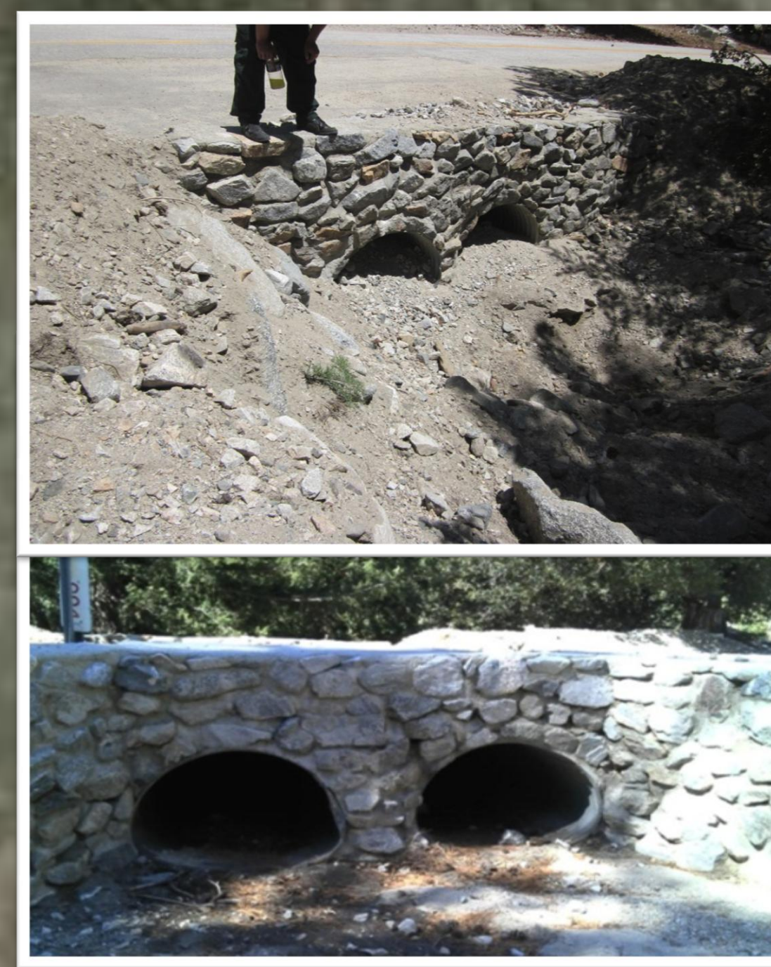
Figure 2: Culvert at point C showing excess erosion and deposition of sediment
