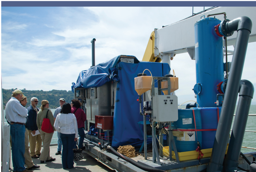
GBF team members and representatives of California State Lands Commission (California's lead ballast water regulation agency) view open-deck installation of the Balpure™ ballast water treatment system on T/S Golden Bear . Image courtesy Lynn Takata, CSLC.
