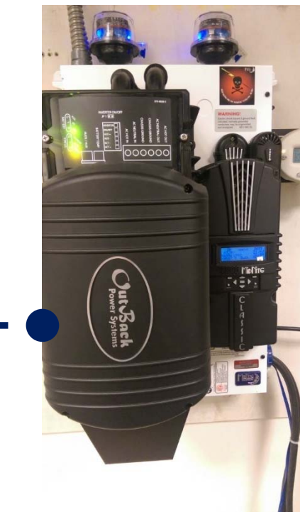
Existing Battery Charger/Inverter System
