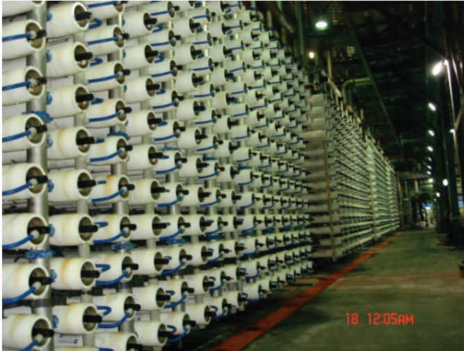
Figure 26. Membrane bank in a desalination plant.
