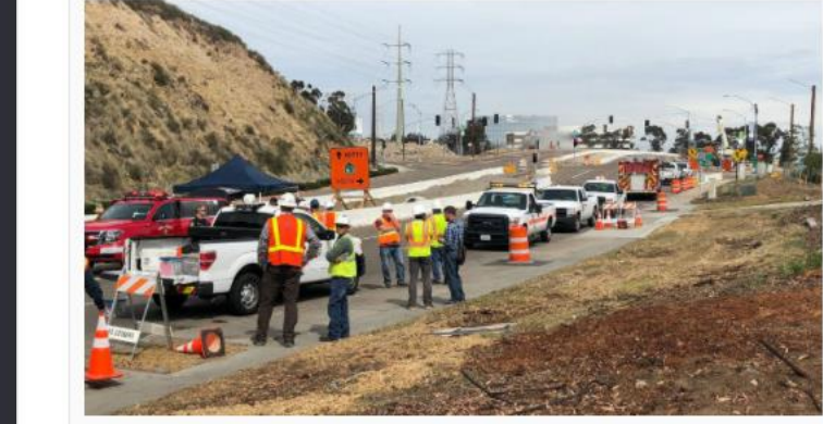
San Diego Gas & Electric crews at the scene of the gas leak. Courtesy SDG&E
