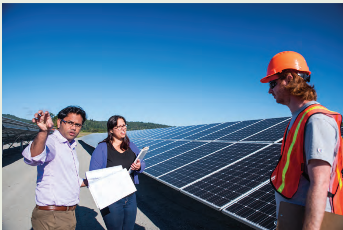
Blue Lake Rancheria Microgrid project developed by the Schatz Energy Research Center at Humboldt State
